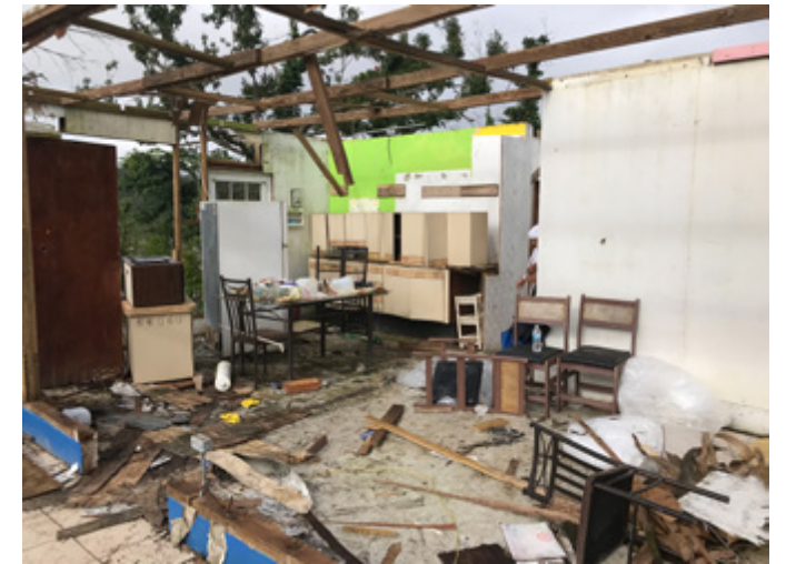
The devastation of a home caused by Hurricane Maria.
